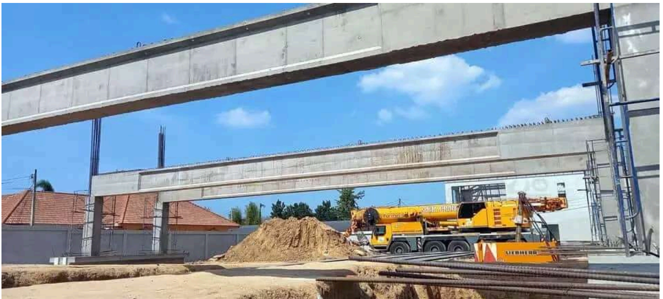
Installation of long-span prestressed concrete girders (up to 30 m) forming the primary structural framework.
